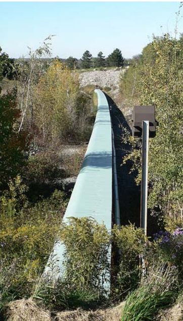
A covered conveyor takes gravel from the source in an Niagra Escarpment open pit aggregate mining operation. PHOTO COURTESY SIGHTHOUND/FLICKR
